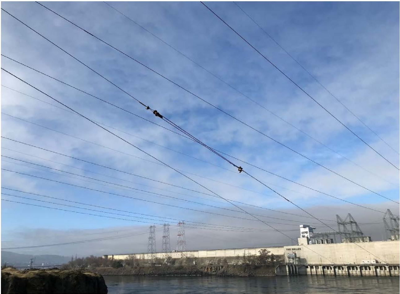
Non-conductive section added to powerhouse avian line array to eliminate shock hazard.
